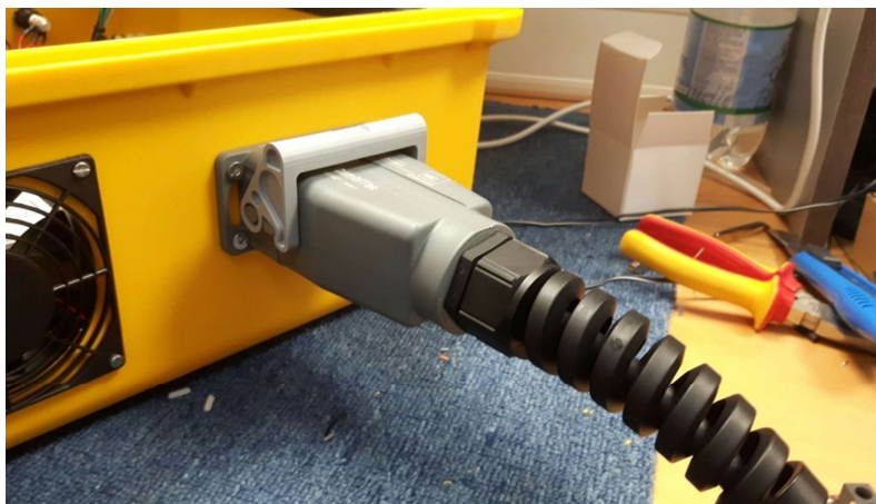
Figure 29: Connection established to the IPG800
