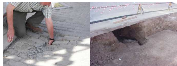
Fig. 1: Nearly outcropped cavity on main road (left) and cavity found during excavations (right)
